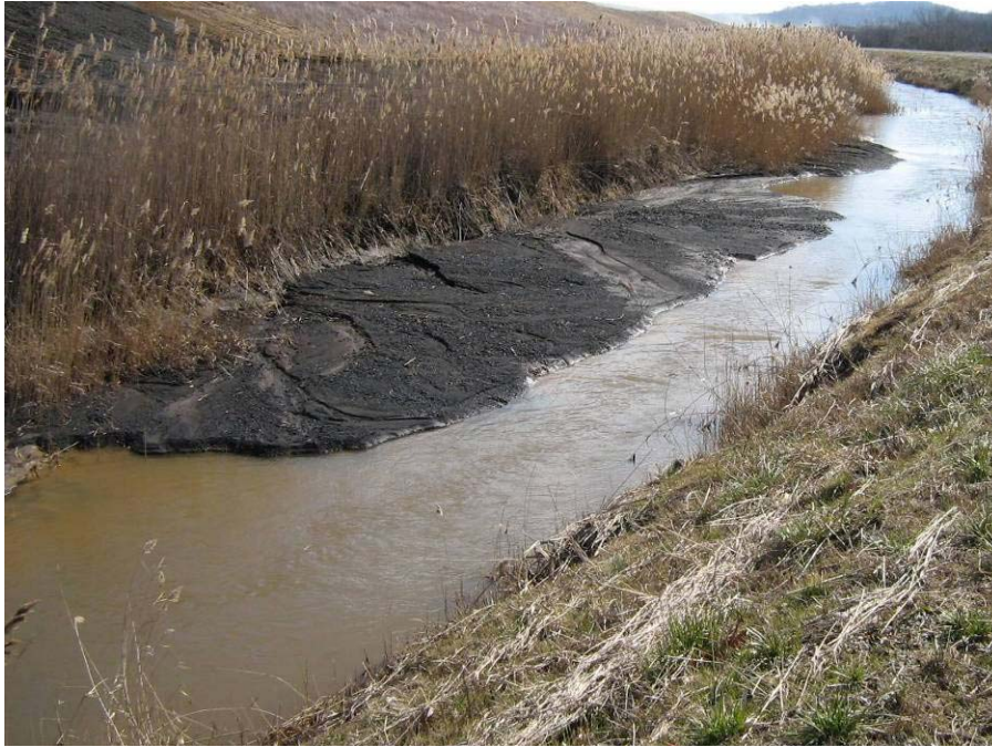
Drawing Mark DS-1-1 Eroded ash from the adjacent dry stack deposited within the west perimeter ditch.
