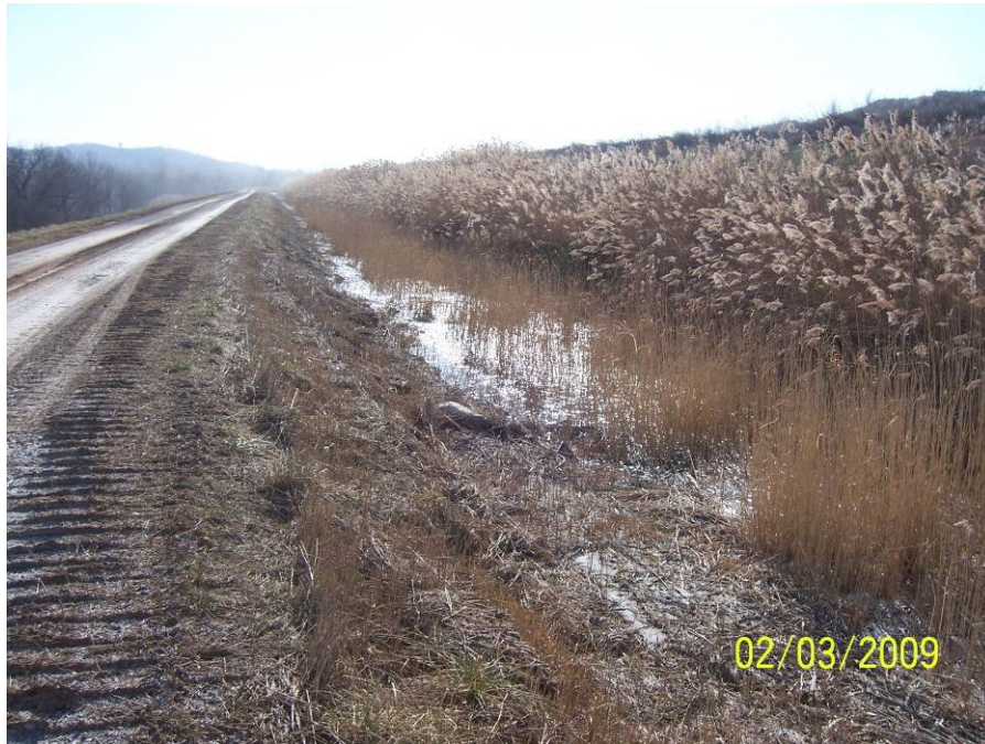
Drawing Mark GP-1-5 Heavy vegetation and sedimentation in perimeter drainage ditch along the southwest and southeast sides of the Gypsum Stack.
