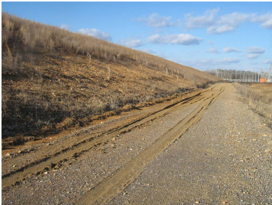
Drawing Mark DS-1-4 Exposed soil and erosion along southeast face of Dry Ash Stack.
