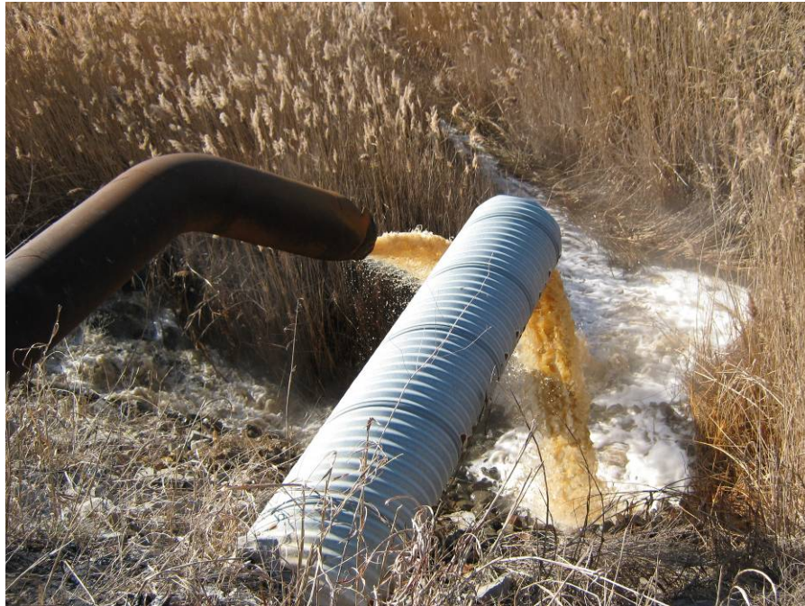
Drawing Mark GP-1-7 Discharge pipes and riprap channel along northwest corner of Gypsum Storage Area.
