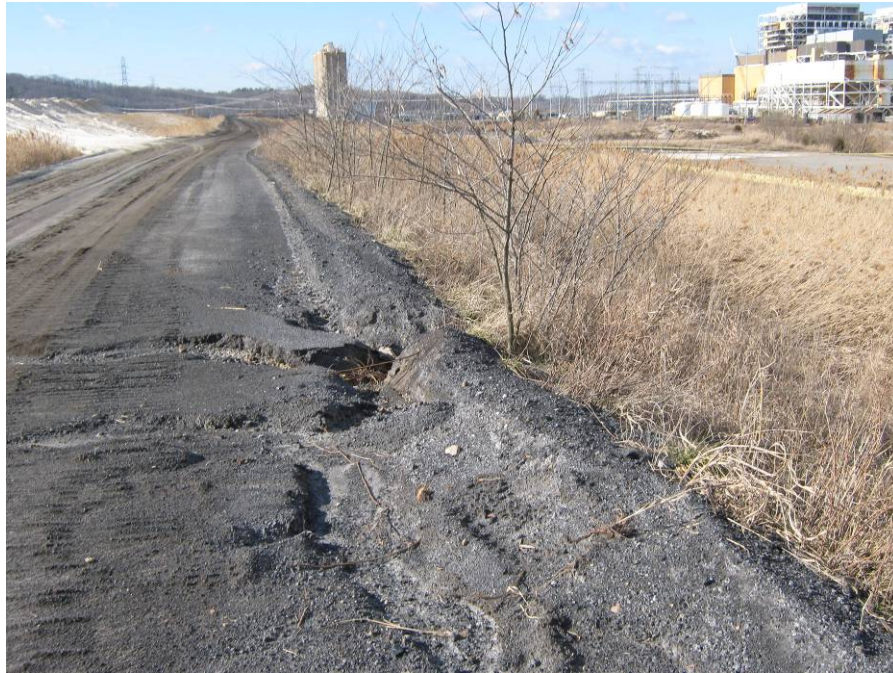
Drawing Mark GP-1-3 Trees and erosion along the perimeter ash dike at the northeast side of the Gypsum Storage Area.
