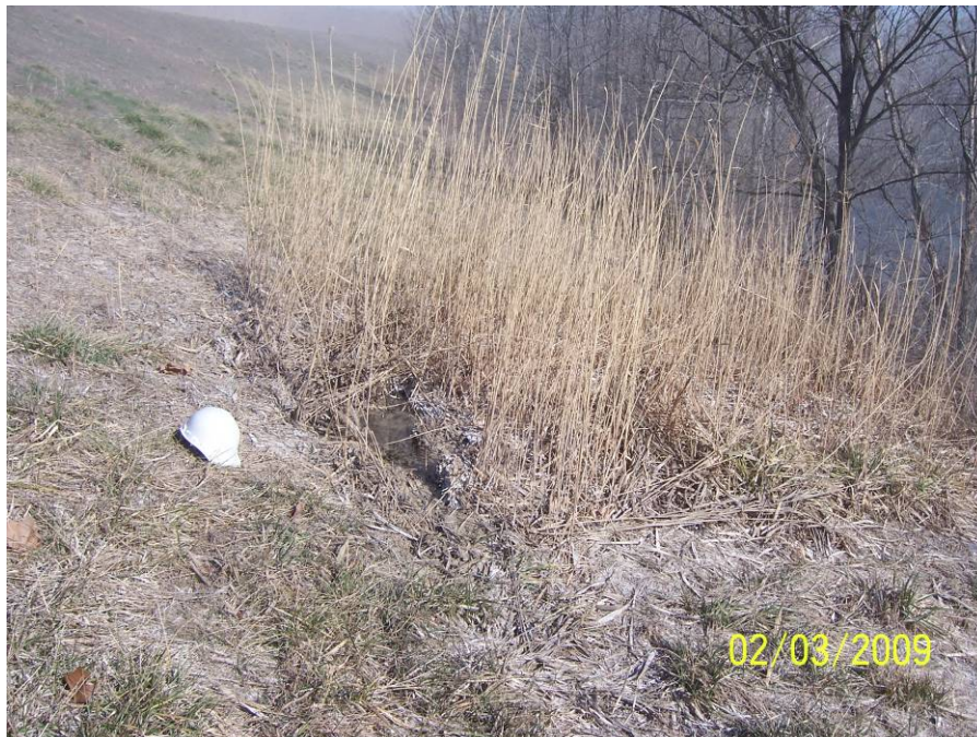
Drawing Mark GP-1-6 Seepage observed below the perimeter dike along the southeast side of the Gypsum Stack.
