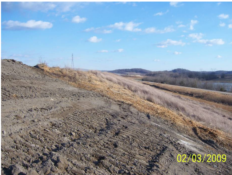
Drawing Mark DS-1-6 Uncompleted soil cover and vegetation along north end of Dry Ash Stack.
