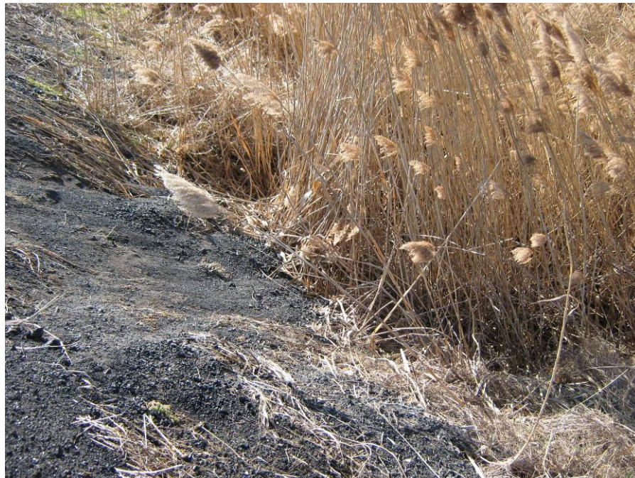
Drawing Mark GP-1-2 Small slope slough along ash divider dike outslope at NW side of the Gypsum Storage Area.
